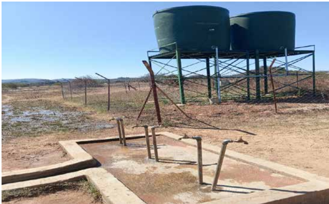
Solarised Borehole, Makoni RDC
