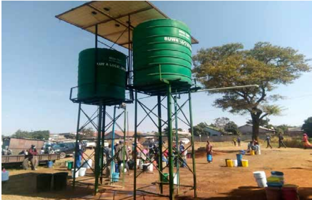
Solarised Water Boreholes, Ruwa Local Board
